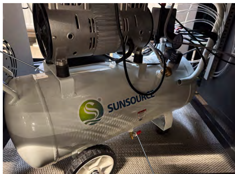
Valve for drainage
